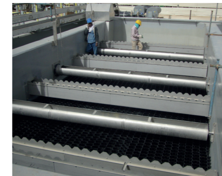
Primary sedimentation with floating material launders
