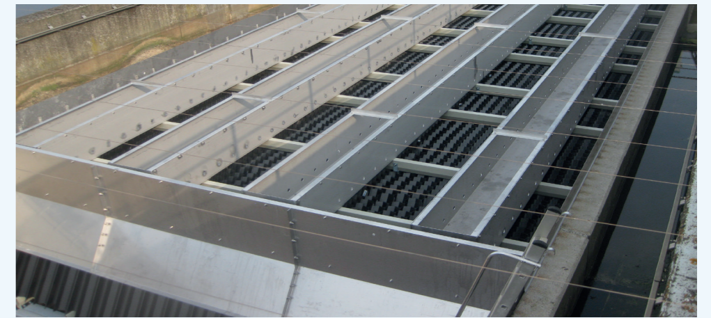
Secondary sedimentation tanks Activated sludge plant
