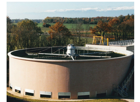
Secondary sedimentation after biological fixed beds – combination of trickling filters and lamella separators
