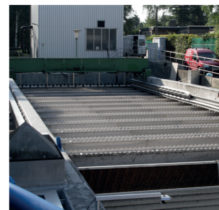
Rainwater treatment plant for 2m³/s
